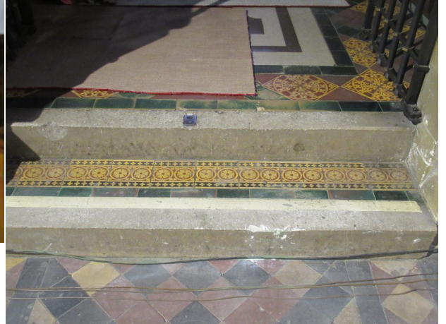
One can now see the step that was covered by the platform at the entrance to the chancel. Note the row of Minton tiles. These same tiles appear along both sides of the nave at roof level.
